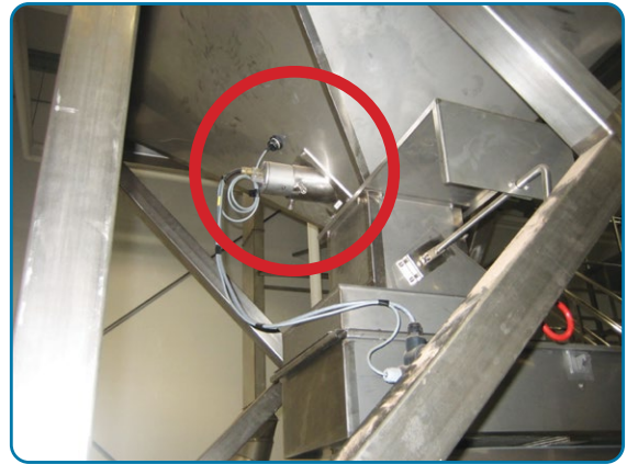
Figure 3: Hydro-Probe moisture sensor installed in the neck of a bin to check the moisture content of the almonds before being released for packing
