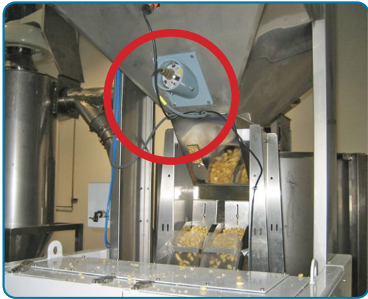
Figure 2: Hydro-Probe installed above a scanner after the dryer enabling real time dryer control
